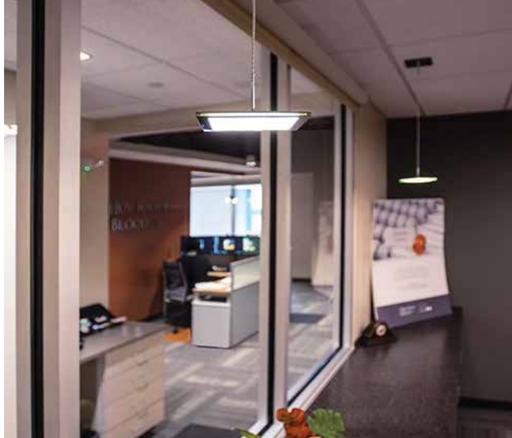
Biorot Zhen single-panel OLED pendant installed at the DKB office
